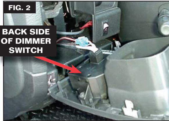
For power to your light, tap into the dimmer switch.
